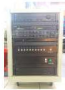
Public Address System (PA System)
